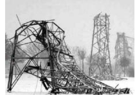
Broken Electric Pylon near Münster, 2005
